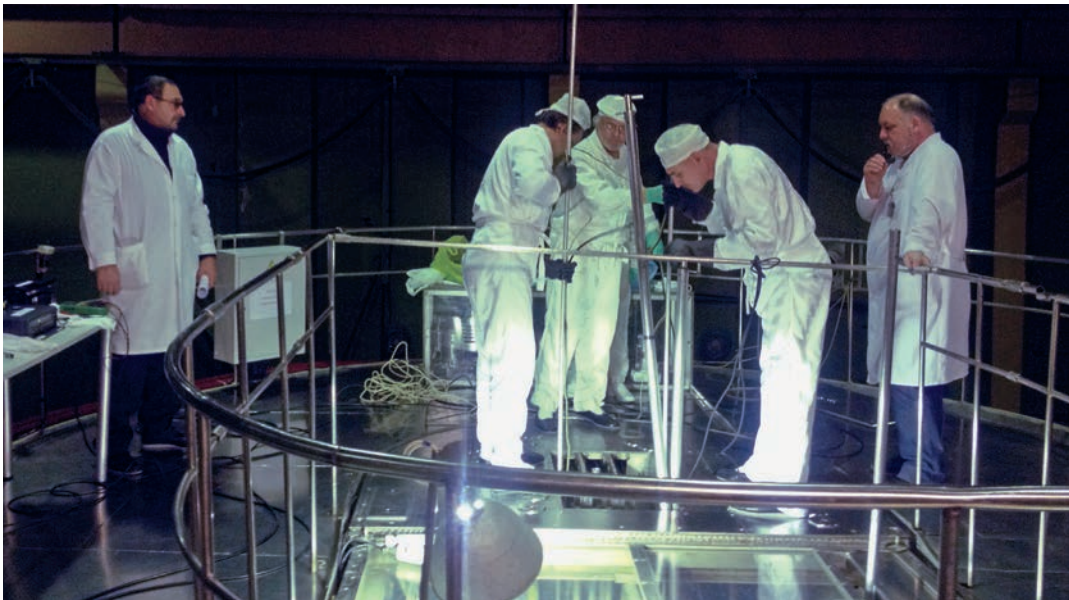
Radiological inventory during decommissioning of the EI-2 reactor at the Production and Demonstration Centre for Uranium-Graphite Reactors JSC (PDC UGR) in Seversk, Tomsk region, Russian Federation (image courtesy PDC UGR)
