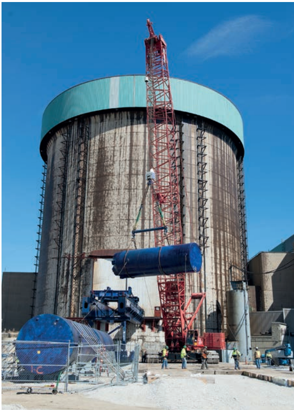
Removal of steam generators during decommissioning of Exelon's Zion nuclear plant. Decommissioning commenced in 2010 and is being carried out by EnergySolutions subsidiary ZionSolutions – see Section A7.1.2 in Appendix 7 (image courtesy ZionSolutions)
