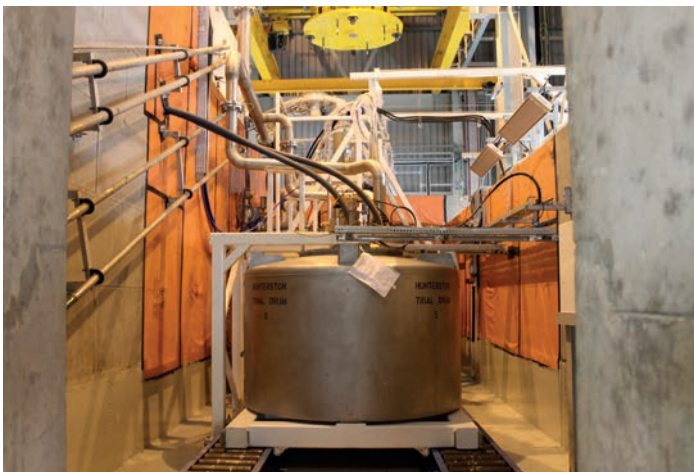
The Wet ILW Retrieval and Encapsulation Plant (WILWREP) at the Hunterston A plant in Scotland. Wet ILW is placed in stainless steel drums and encapsulated with cement prior to storage for several decades (image courtesy Magnox Limited)
